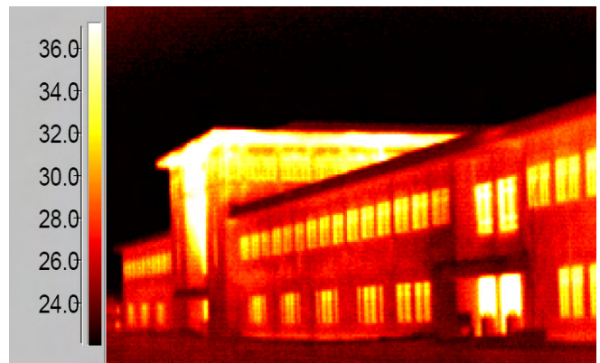
Image 11: During the commissioning of this building thermography revealed an extreme problem involving exfiltration through the soffit. Courtesy Phil McMullen.
