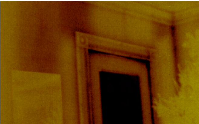
Image 4: Properly installed cellulose is an excellent insulation. Unfortunately, it is often poorly installed with missed areas and settling the most common quality problems.
